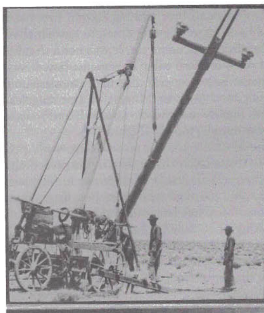
Figure 3.2 Line crew with horse drawn wagon erecting a transmission pole in the desert with a derrick and gin pole, California ca. 1903. Reprinted courtesy of The Huntington Library and the papers of Southern California Edison.
